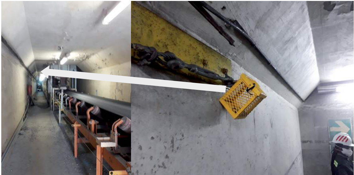
Figure 8: A rod mill tunnel (left) – the arrow shows the location of the monitoring equipment close to rear of tunnel.
