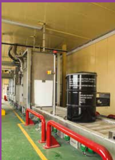
The recently installed drum-filling machine.
