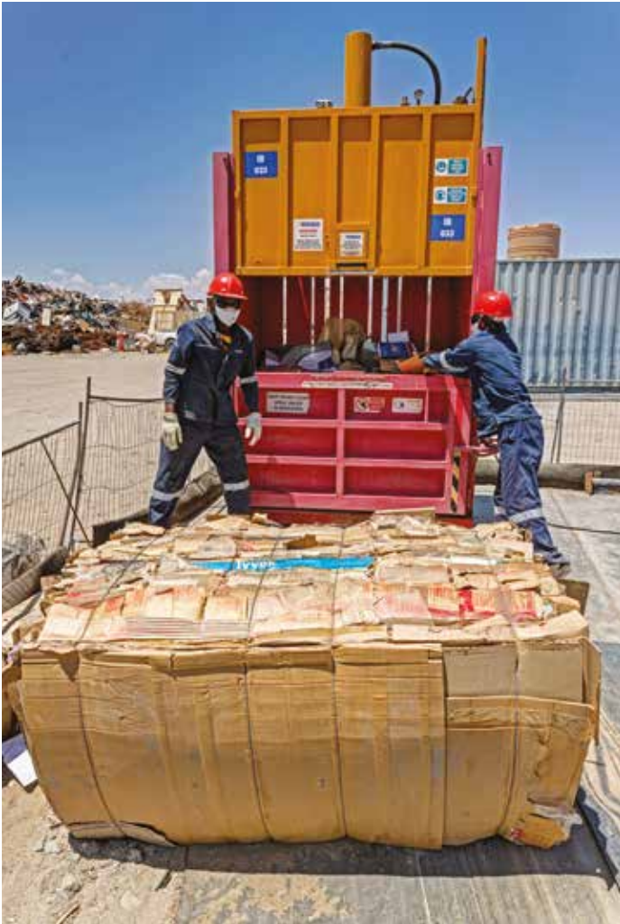
Two bailer-machine operators of Rent-a-Drum, the waste management contractor appointed to handle recyclable materials such as scrap metal and packaging materials onsite, are compacting packaging material.
