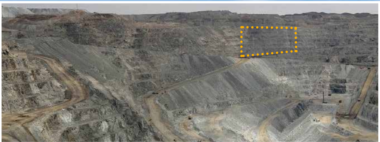
(Inset photograph) The yellow dotted lines indicate the Trolley 14 area of the Open pit where the drape wire meshing was installed to eliminate rock fall.
