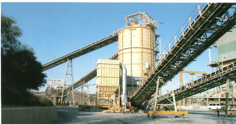
DUST: A new dust collector was installed at the pre-screening plant and is one of many control points to monitor dust on site.
