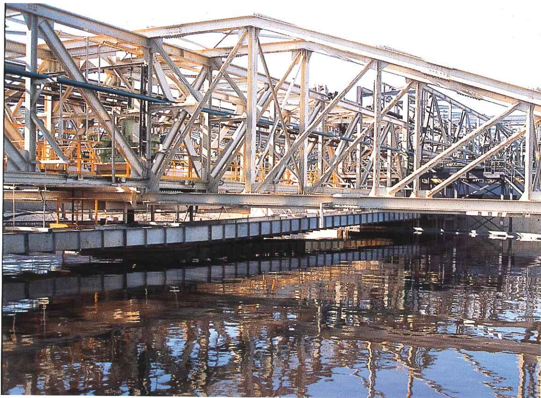
Counter Current Decantation Thickeners
