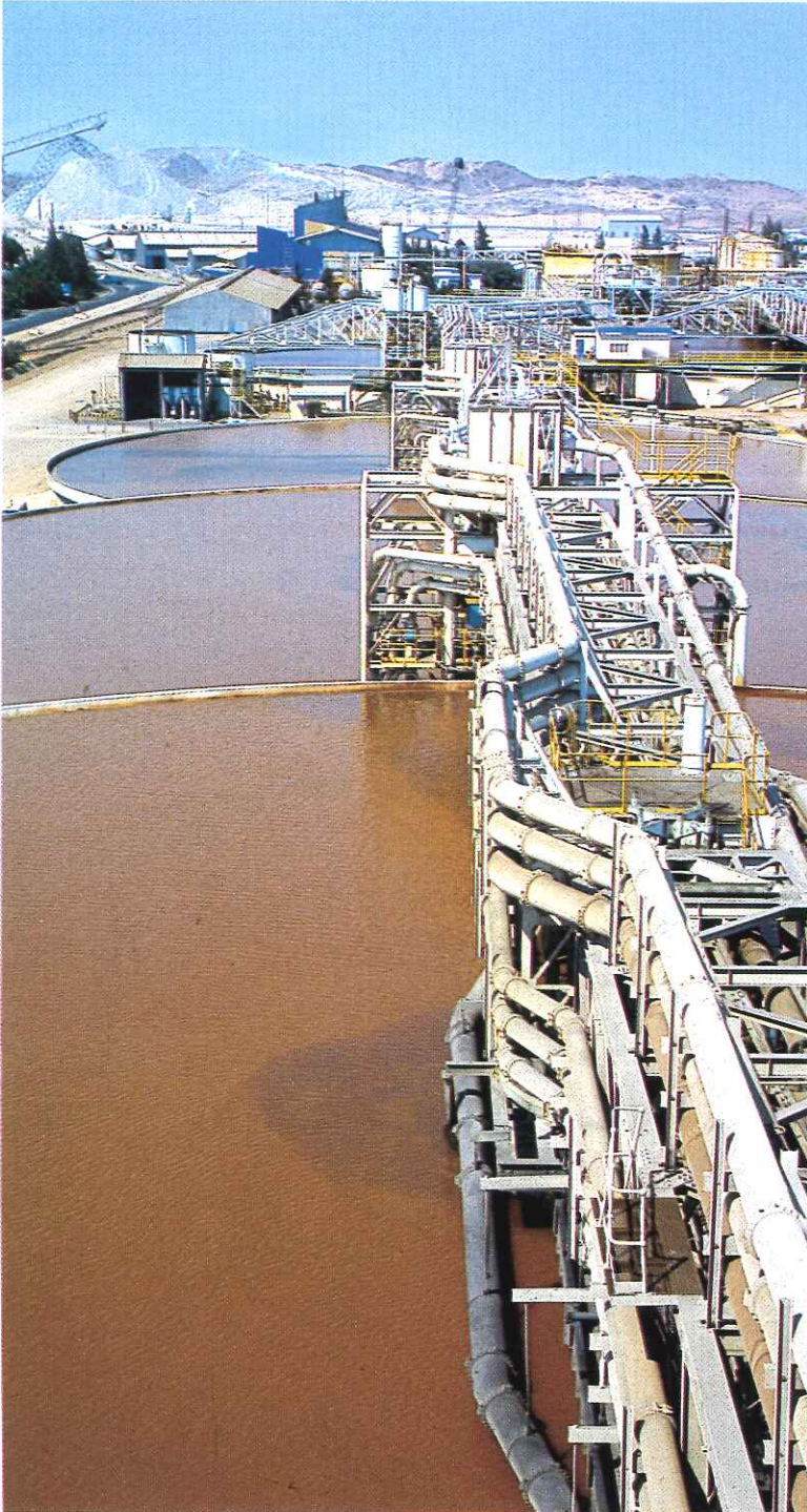
Counter Current Decantation Thickeners
