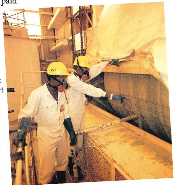
Inspection of a rotating drum filter in the final product plant.
