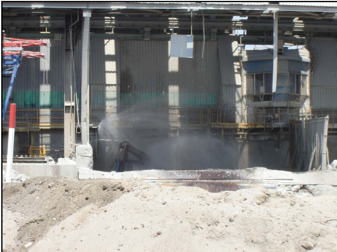
Figure 4-10: Water sprayers at the primary crusher to reduce emissions of fugitive dust due to off-loading operations (i.e. materials handling operations)
