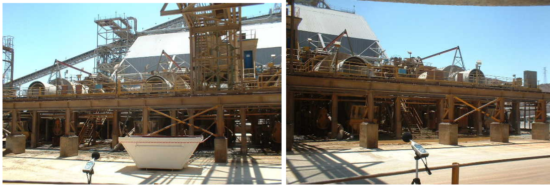
View of the Rodmills, two to the left and two to the right of the centreline
