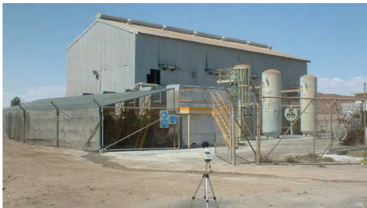
Compressor House and Cooler Bank
