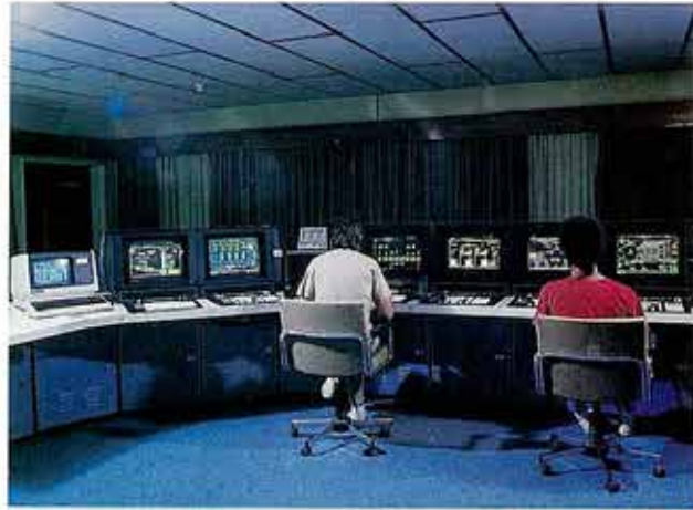
(A) The computerized Central Process Control operates the metallurgical plant.
